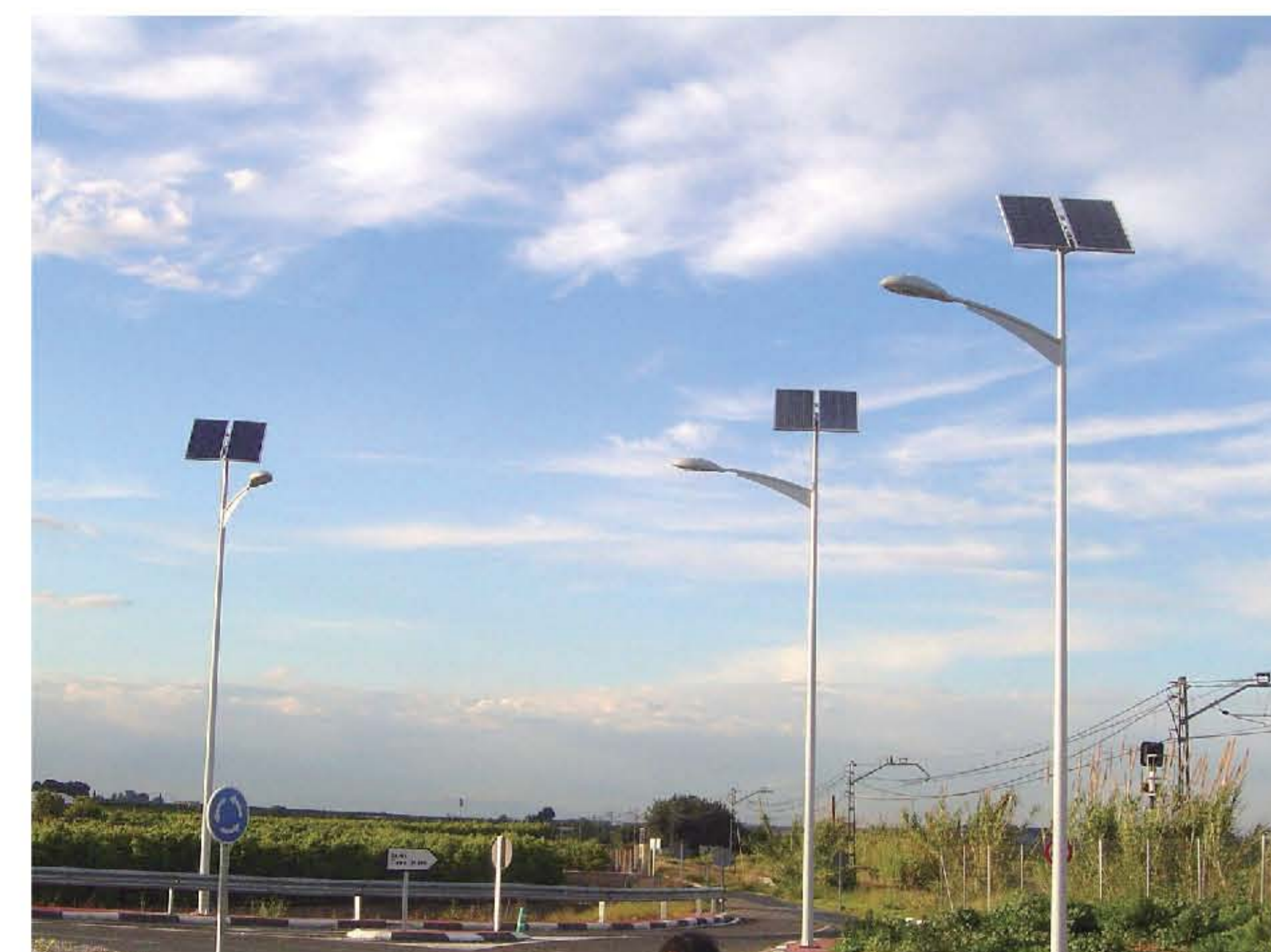
Solar street lamp in Spain
